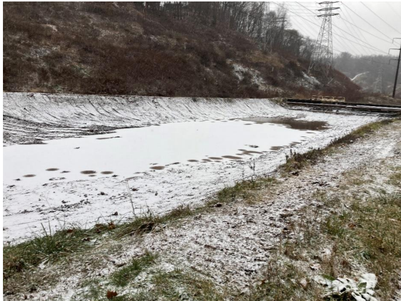
Photograph 3: Bottom Ash Recycle Pond, facing Northwest. Date: 12/16/2020 Description: Bottom Ash Recycle Pond following CCR removal.
